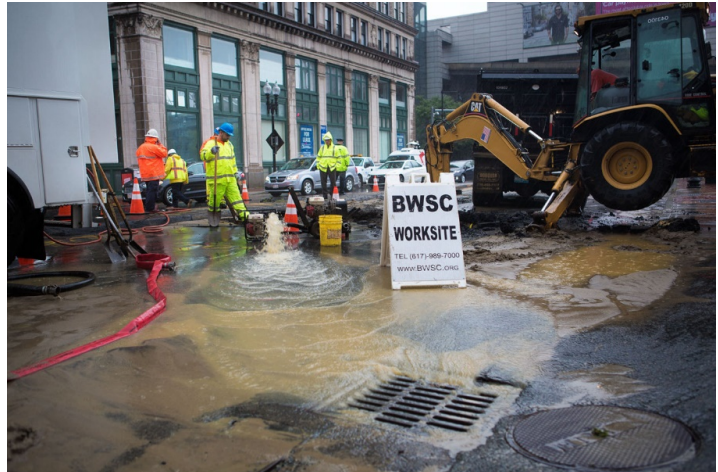
Water main break in downtown Boston.
