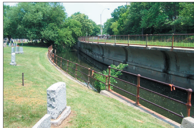
FIGURE 61. On the east side, a concrete retaining wall with a cantilevered sidewalk defines the brook’s edge in the Parkway section between Henderson bridge and Broadway.
