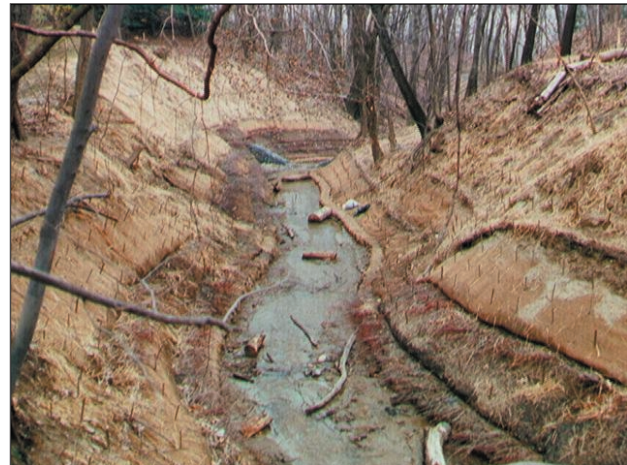
FIGURE 24. This stream channel is being restored using bioengineering techniques. These techniques, originally developed in Europe, combine mainly natural materials such as native plants, coconut fiber mats, and rock. They have proven very successful in restoring natural systems.
