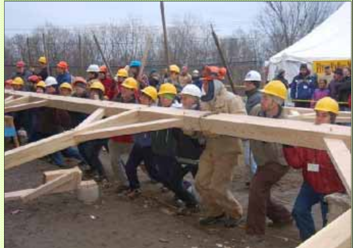
Community raising of a timber frame for a new food cooperative (HomeGrown Wood™ hemlock and locust), River Valley Market, Northampton, MA.
